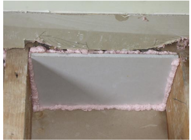
Fully 'buttering' a suitable sized piece of board with bonding plaster or even with fixing foam and sticking it to the wall can be suitable for sealing gaps in the floor void walls.
