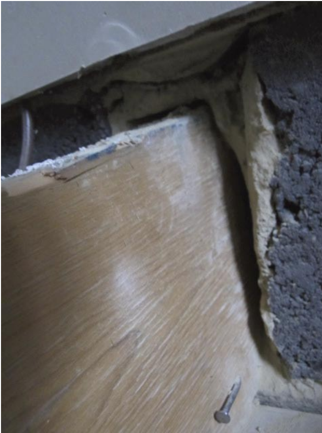
Building works are rarely properly sealed off behind dot and dab dry walling as the pictures here indicate.
