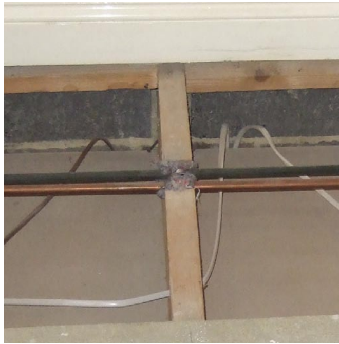
Cable runs and entries can allow draughts to enter and circulate. These can be safely sealed with acrylic sealant. In new homes or on rewiring this should be done routinely.
